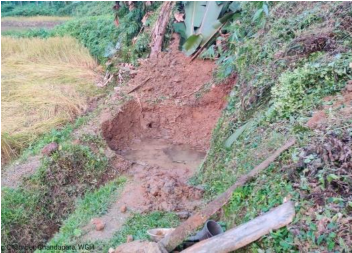
BEFORE- Construction of Spring Chamber started at Jongsin Gittim, Chandapara, Dalu Block, WGH 23.11.19
