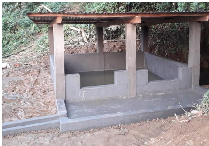
Spring Chamber at Sombalin Chiga, Chandapara as on 7th Jan 2020
